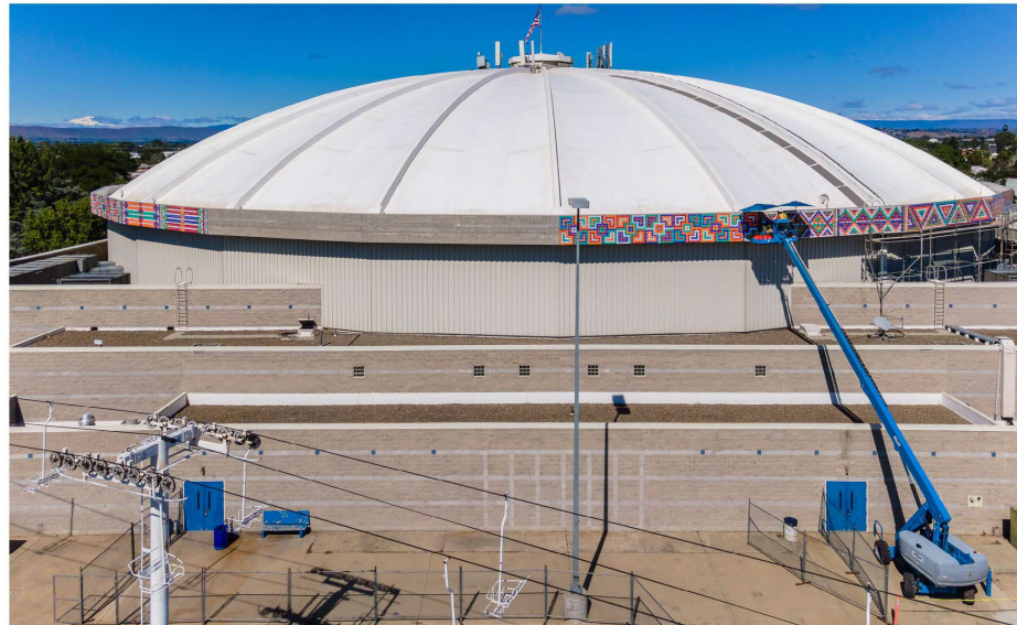
ArtsWA's restoration contractors use a bucket lift to reach the damaged panels. Photo by Yakima Valley Photography.
